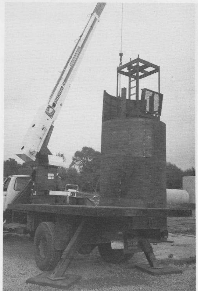
Fig. 3. Assembly of concrete form and 3 deck scaffold on surface. Assembly includes a pair of guides and guide brackets to ensure an exact fit of all components and to train crews in their use.
